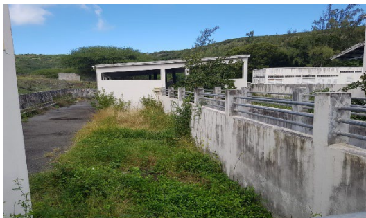
Figure 11: Yard and buildings left in abandoned state
