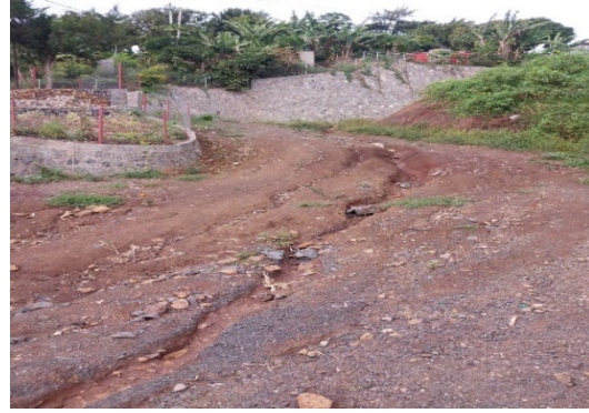
Figure 7- Natural drains along access road far from retaining wall
