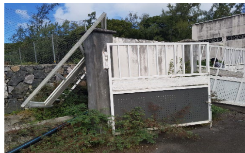
Figure 12: Detached metal gates
