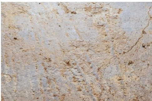
Figure 2: State of the flooring
