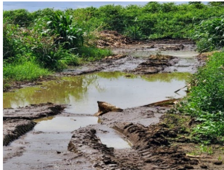
Figure 1: Condition of the track road
