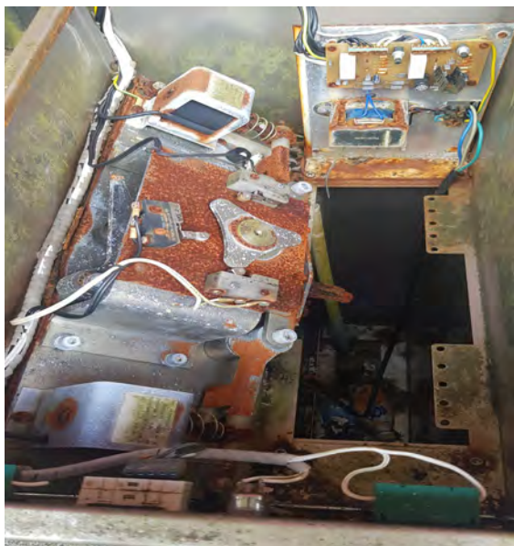
Figure 8 Electric Wire Exposure at Entry Gate of New George V Stadium
