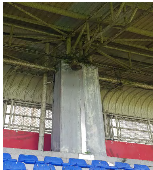
Figure 9 Damage to Bird Nets and Surveillance Camera at New George V Stadium
