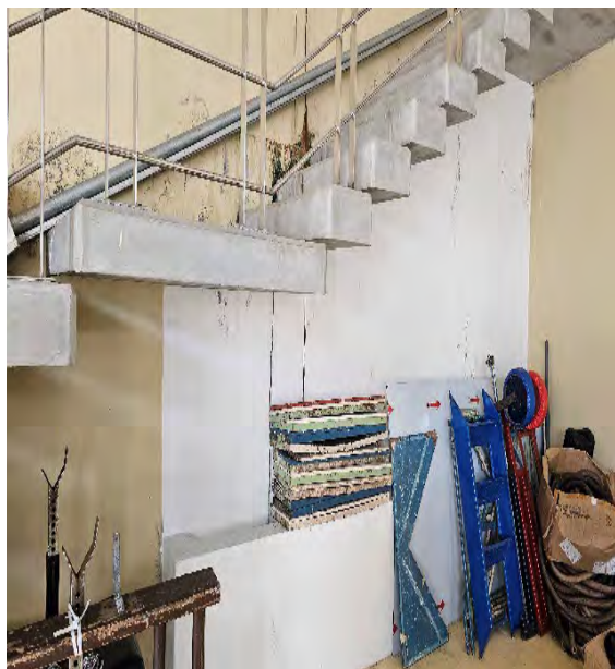
Figure 10 Water Leakages on Wall of Gymnasium at Vacoas Sports Complex
