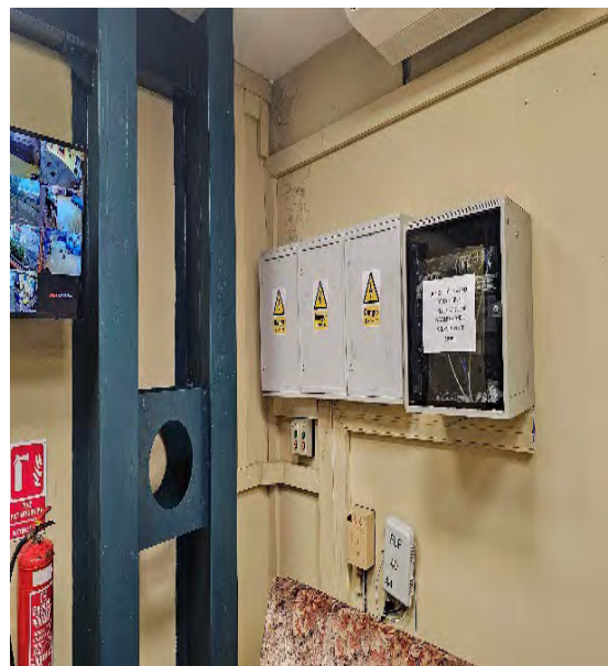
Figure 11 Water Leakages near Electric Panel at Vacoas Sport Complex
